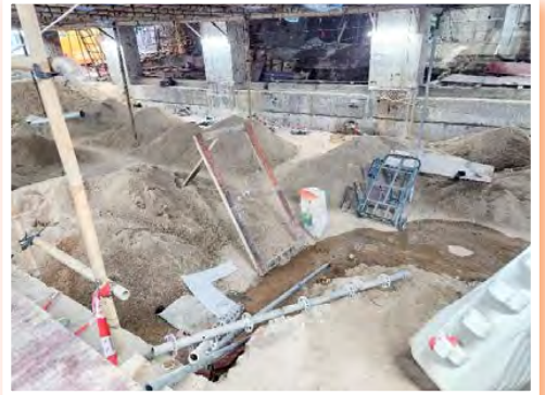
Indoor Swimming Pool with backfill material for use upon laying of pipe works around the pool.
