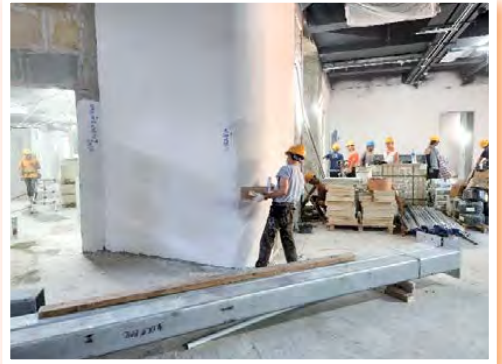
Skim coating to block wall at the interior of the Main Entrance
